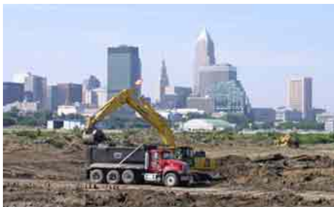
Dredged sediment from Dike 10B near Burke Lakefront Airport being removed and transported to remediate a Cleveland Brownfield site.
